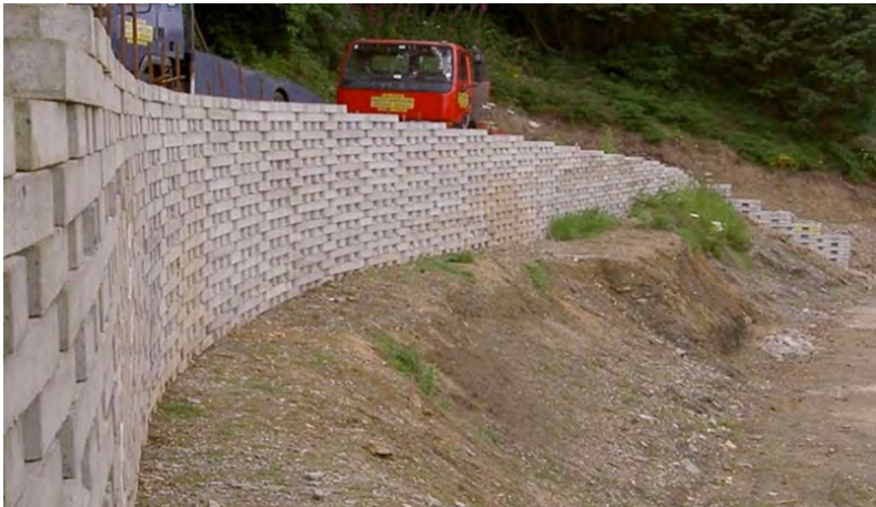
Aqacast highway and river protection retaining wall
