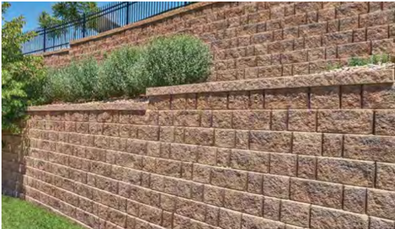
Keystone retaining wall
